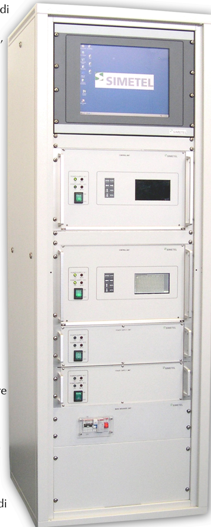
Rack with two control units, two power supply units, one control panel.
